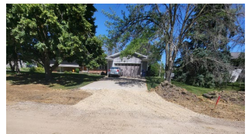
TEMPORARY ROCK INSTALLED IN DRIVEWAYS AFTER BEING CROSSED WITH NEW STORM SEWER
