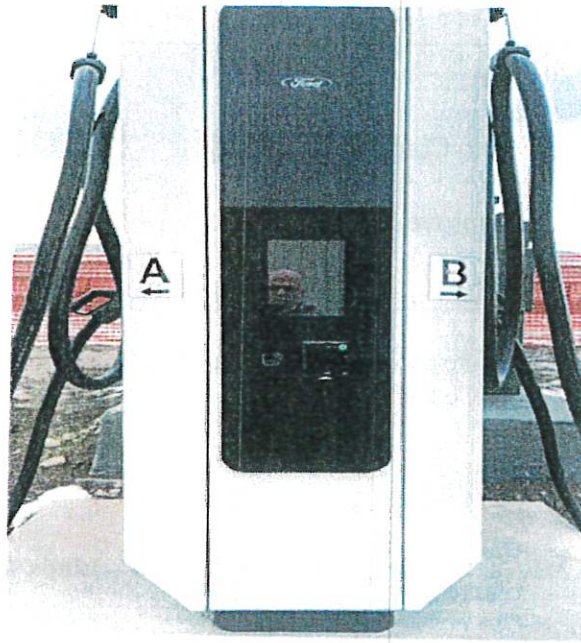
O'Rourke Ford Motors After photos of Charging Station Project
