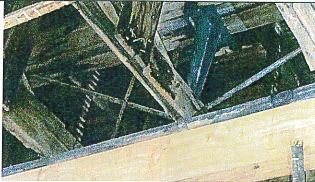
Photo 9 | Grid B Inverted King Post Truss with Underhung Ceiling Joist Support Beam.
