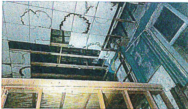
Photo 17 | Second Floor, West Exterior Wall at Center Beam Bearing.
