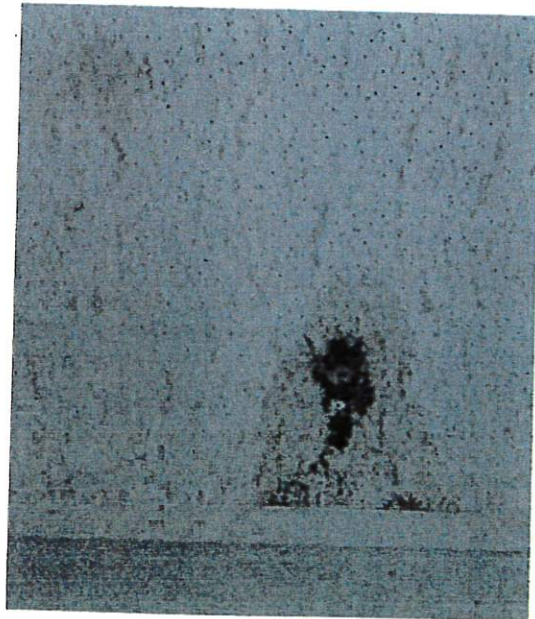
Ceiling water and mold damage
